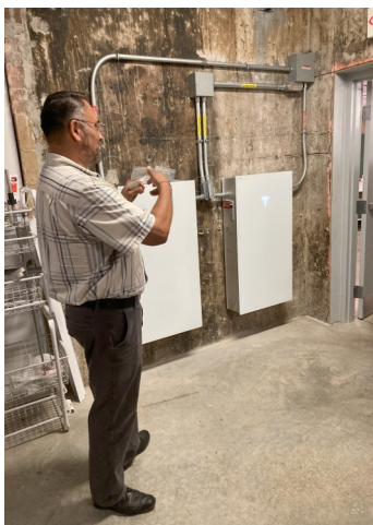
Photo: David Gomez, owner of Daily Green Power, explains operation of Tesla Powerwall batteries at FCCES office.
