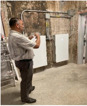
David Gomez discussing the new Tesla Powerwall Batteries installed.
